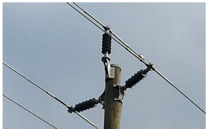
33kV Polymer Posts - Otago
