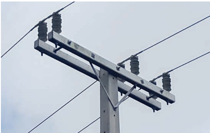
11kV Polymer Posts - King Country
