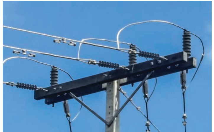
33kV Polymer Posts - Taranaki
